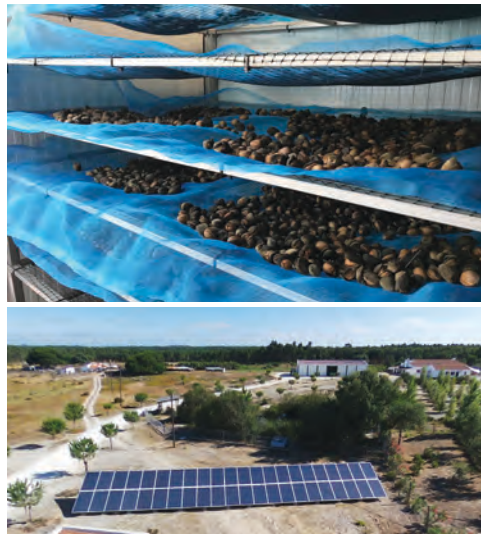
TOP: Solar dryer for local products and PV plant with 44 modules installed.
